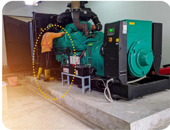
Image source: Vecteezy; https://www.vecteezy.com/photo/7360793-a-technician-is-doing-regular-maintenance-on-the-generator-engine
